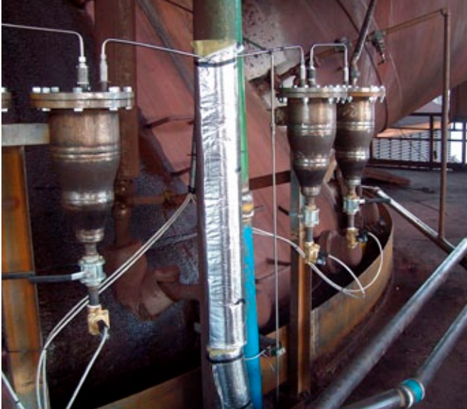
Dust / moisture pot on sampling lines from off-takes
